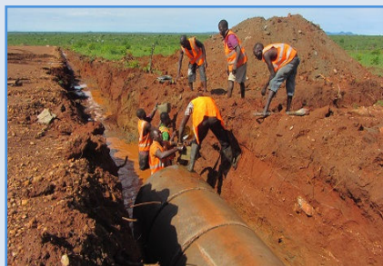
Heavy rain constrained culvert work by flooding the culvert—PoC 3, Juba
