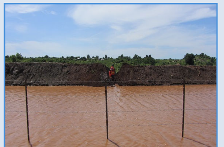
Flooded sections of the internal and external road after the rain on 21 May—PoC3, Juba
